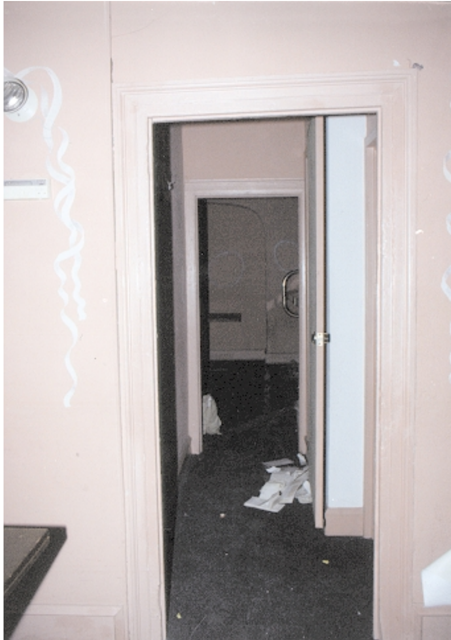
Second floor view from north room through entry hall (original door trim) (KAA:97-15/18) 12/6/97
