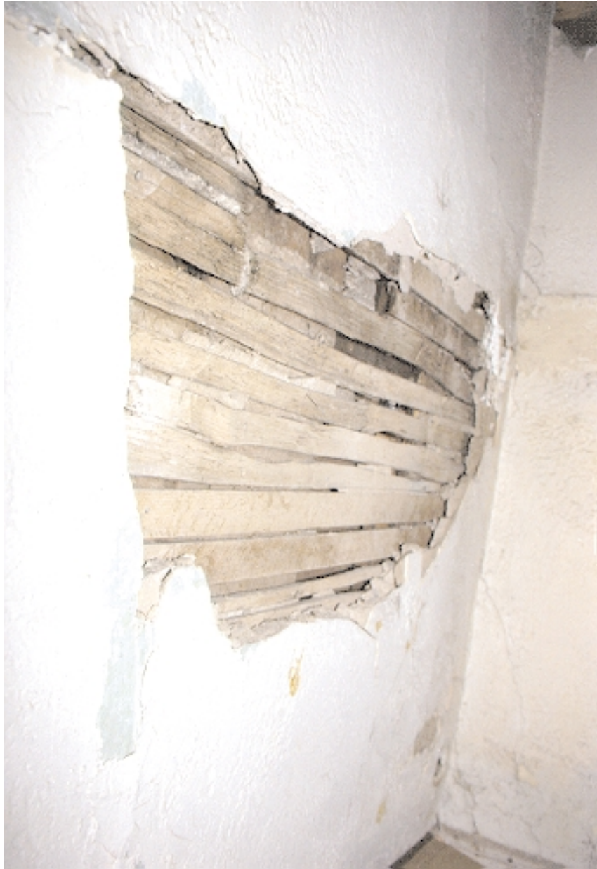
Interior partition wall, stairwell to attic. Lath detail showing both hand split and circular sawn.
