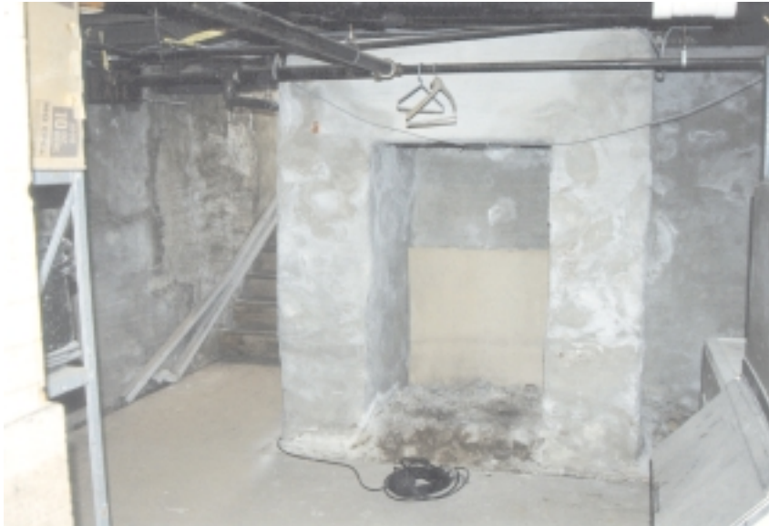
Basement fireplace support, south wall near southeast corner (note entrance to left) (Doug Crompton 12/6/97)
