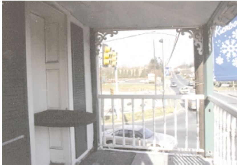
Northeast corner of porch, 2nd floor, original porch railing mortise hole in post. Recessed window openings (KAA:97-15/16) 12/6/97
